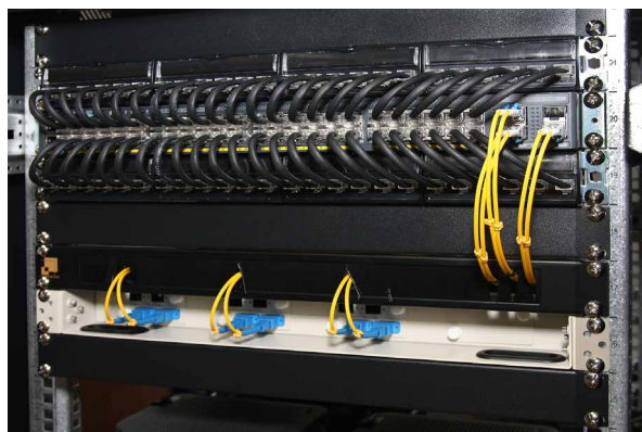
Example of a patch panel with ethernet cables
